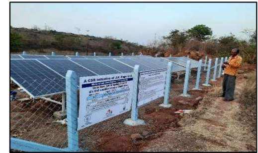
Solar based lift irrigation
