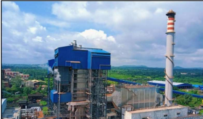
High Pressure –Cogen PP
