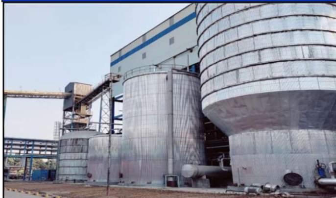
DDS technology digester
