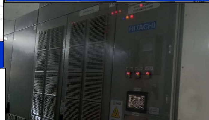
HT VFD for feed Pump
